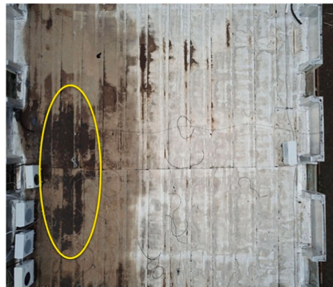
Fig. 4. Reference area for annotating dark stains.
