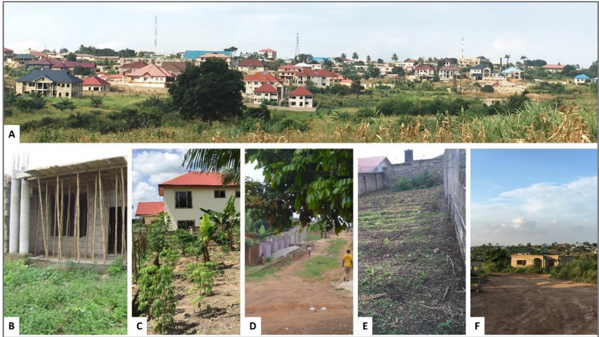
Fig. 3. Field impressions of areas with on-going housing construction that are classified in this study as the urban-open-space. Pictures by S.B. Asabere (Kumasi, Aug–Sep 2016).
