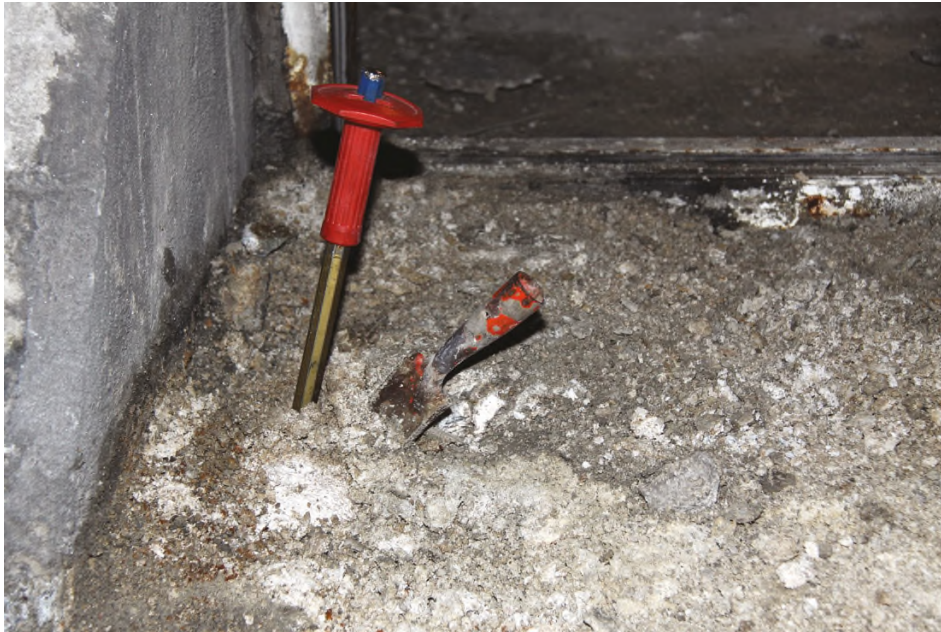
Figure 1: Concrete completely destroyed by intensive thaumasite formation.
